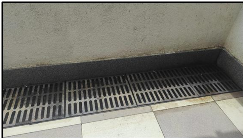
Drainage observed in the campus
