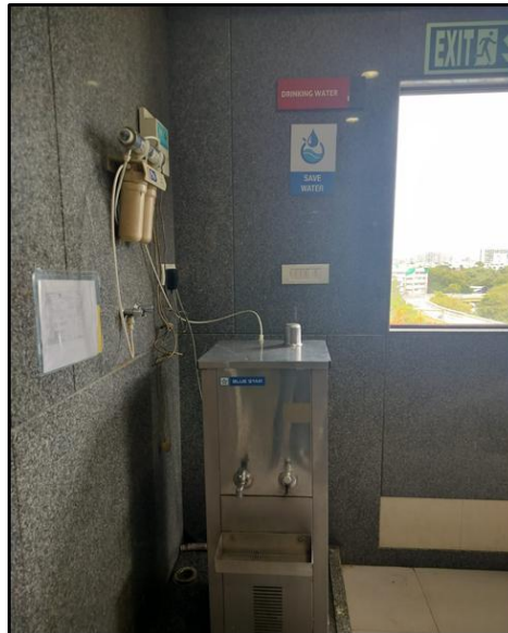
Water supply systems observed in the Campus
