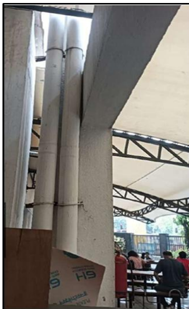
Water Management System observed in the campus
