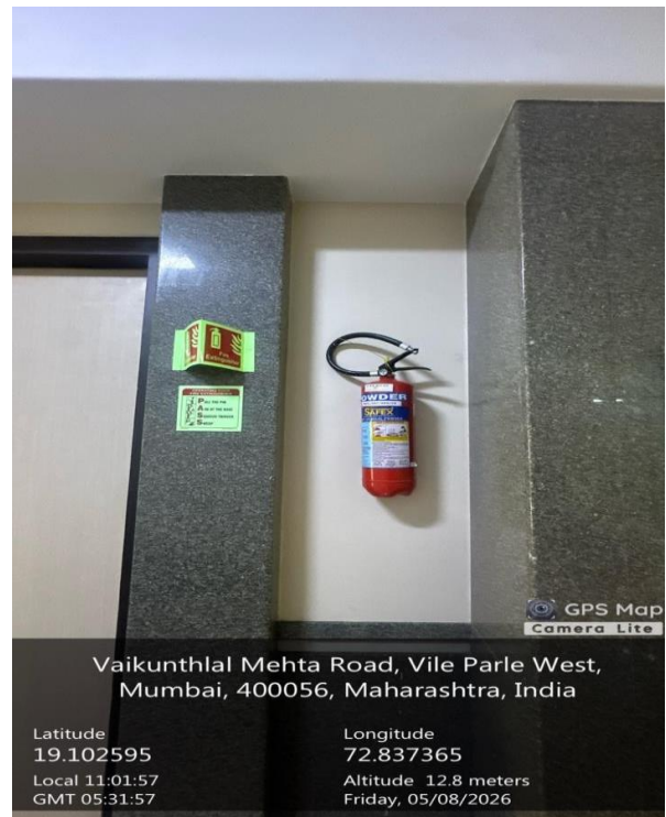
Fire Safety Equipment
