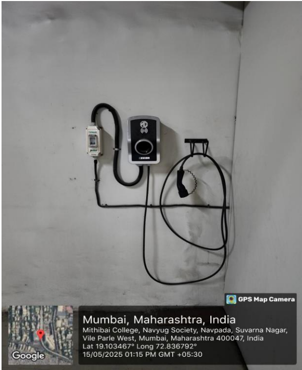
EV Charging Points
