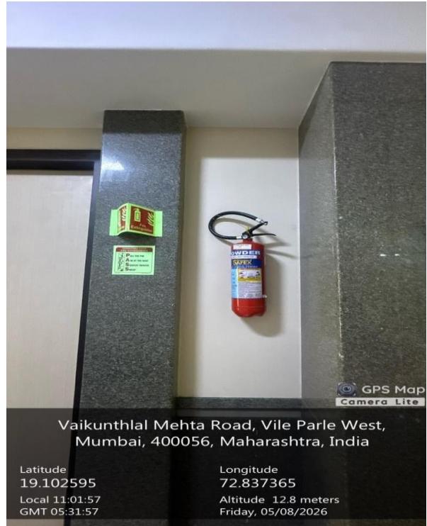
Fire Safety Equipment
