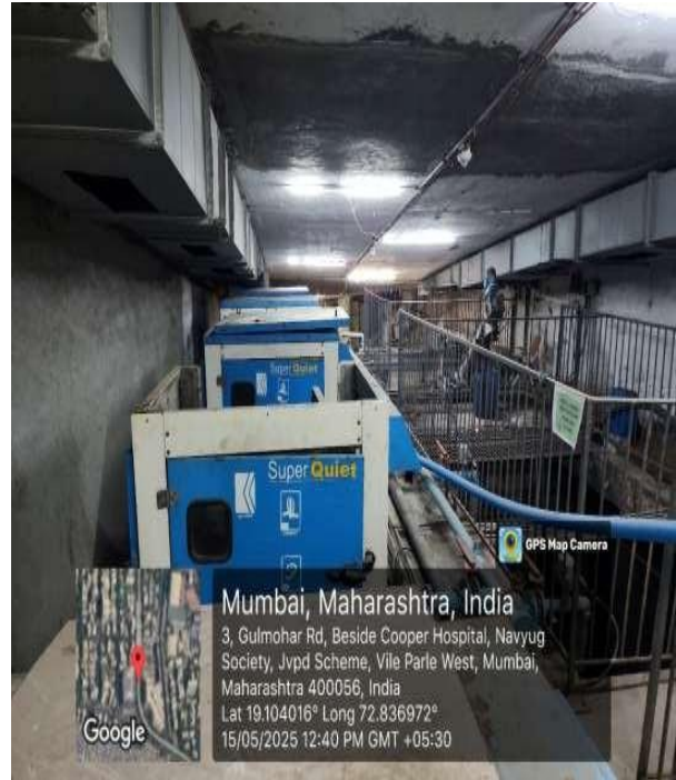
Sewage Treatment Plant
